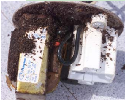
Below: Electrical box short due to RIFA
